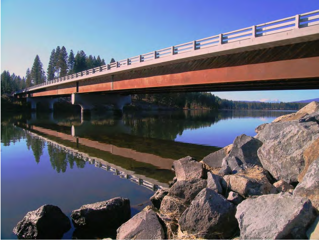
Figure 10-6. Spencer Bridge on State Highway 66 in J.C. Boyle Reservoir. Picture taken from the downstream side east abutment.
